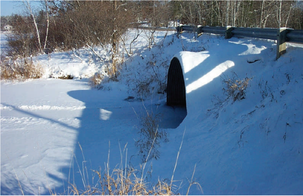
The culvert under County Highway Y near the boat landing is the official Cloverleaf Lakes depth marker. The lake level is measured downward from the top of the culvert and should be between 72 inches and 78 inches, according to DNR records.
